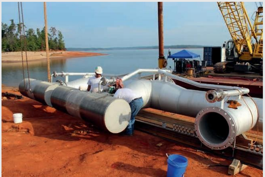
JOHNSON SCREENS® Passive Intake Installation: Drinking Water Plant in South Carolina, USA
